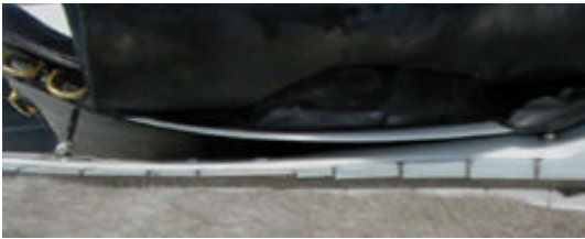
Gap with no packing shims in place
