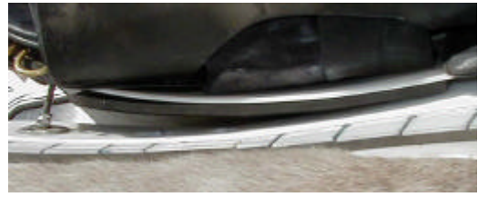
First full length shim in place to ensure contact from bridge to panels
